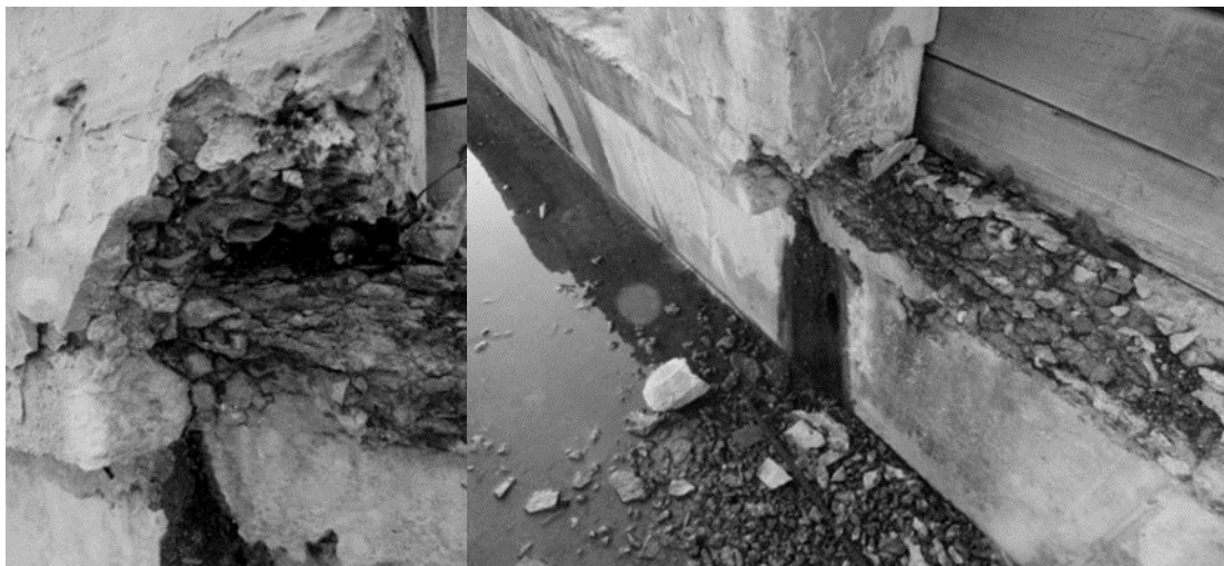
Fig. 1. Corrosion destruction of the reinforced concrete wall
